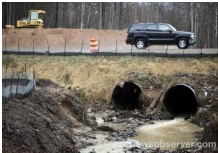
Figure 4-6 Perched culvert (credit: Raleigh News and Observer)
